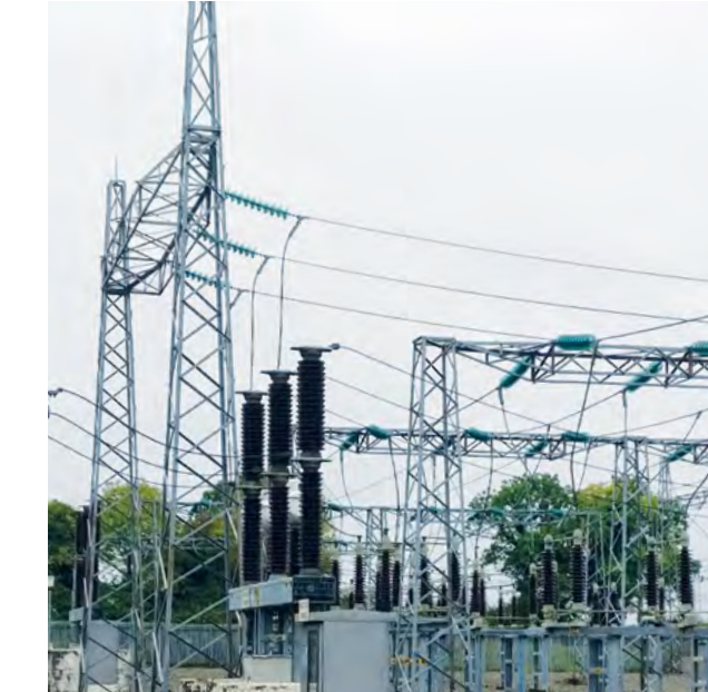
EirGrid Substation, Ireland
